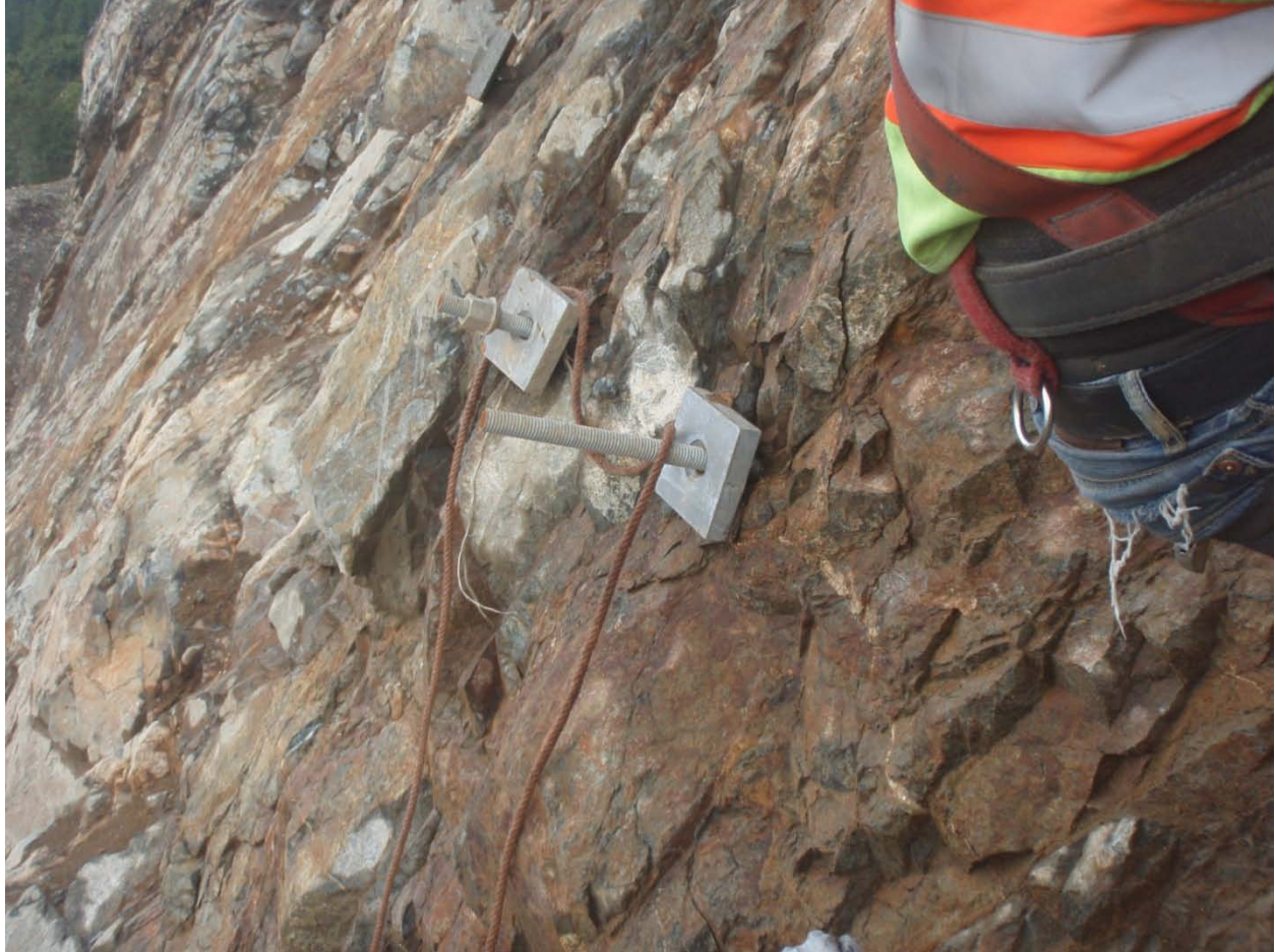
Figure 2. Anchors on Cut 9/Segment 1. Anchors not properly installed. Limited or no grout and anchors not tensioned.
